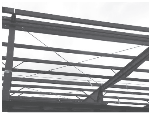
Tie rods are used for cross bracing to stiffen the roof of a building to resist wind loads.
